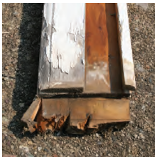
Rotted, Traditional Frame
